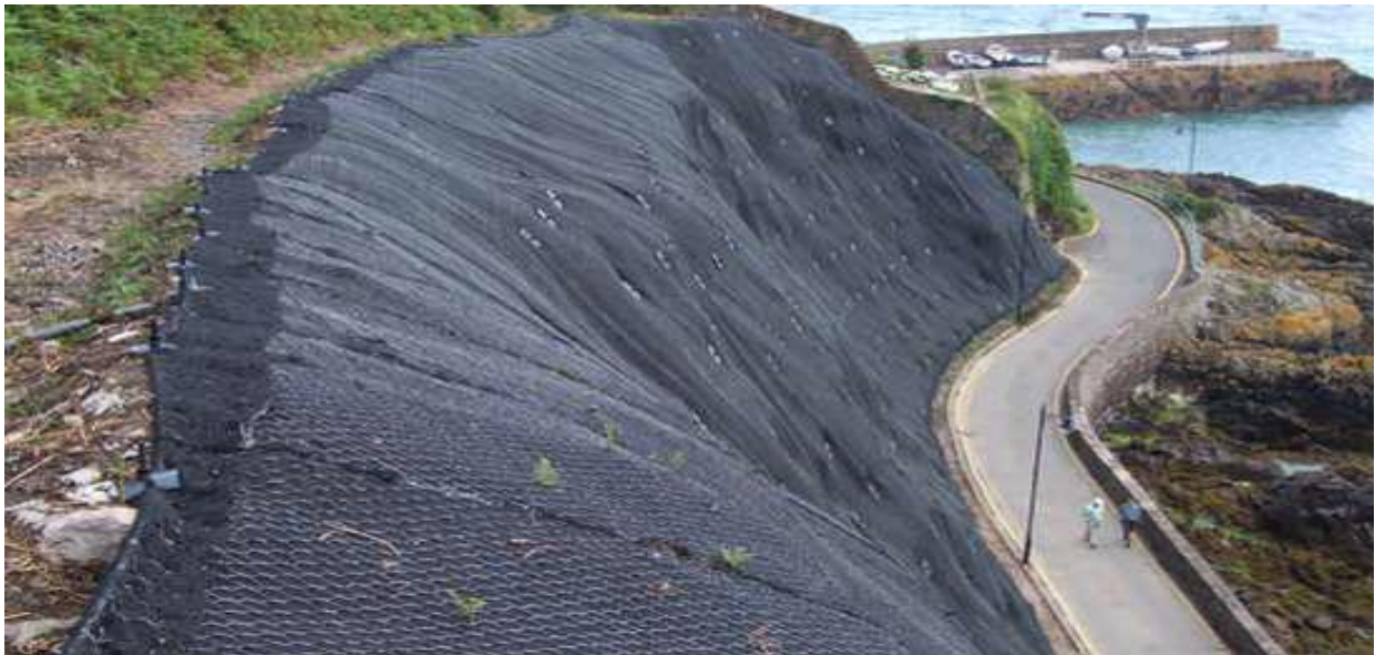
Figure 5. The meshed geo composite bitumen layers for protecting against shear and erosion in flood.
